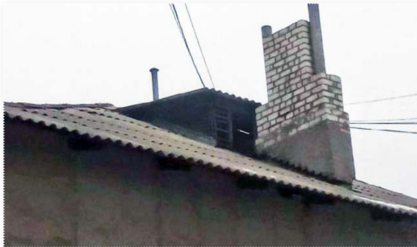
The attic of the house No.381, from where a shot could be made
