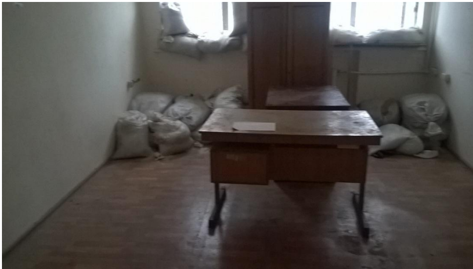
The premises inspected by the members of the monitoring group in the former office building of the Lysychansk glass factory
